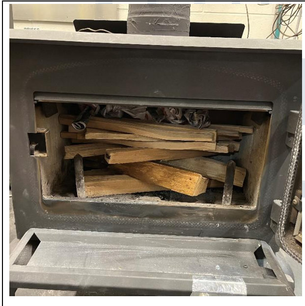
Kindling & Start-up Loaded in Stove
