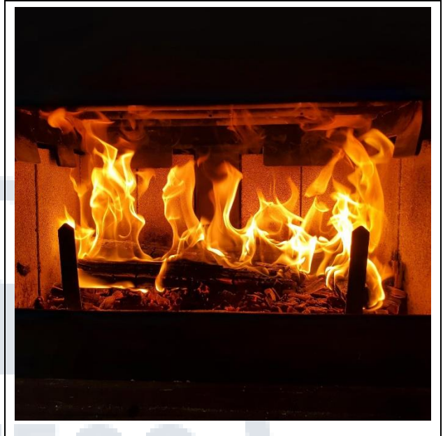
Residual Start-up Fuel Coal Bed – Post Rake
